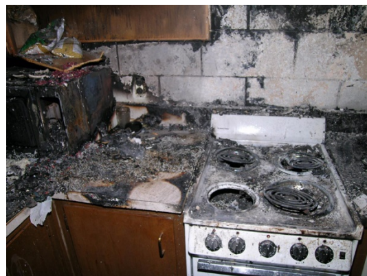
Kitchen fire damage. Source: Seattle Fire Department
