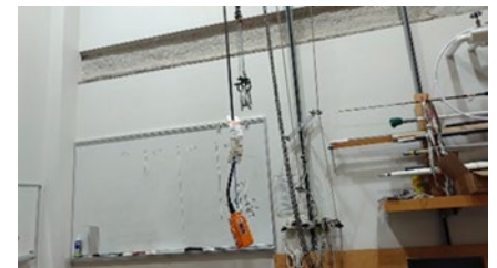
Figure 13: Pendant Controls (UW installation)
