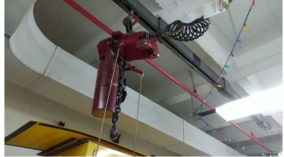
Figure 11: Air - Pneumatic hoist (UW installation)
